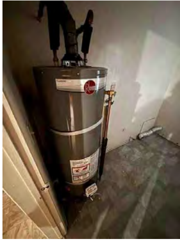
5034 West Slauson Ave. - Water Heater Double Strapped
